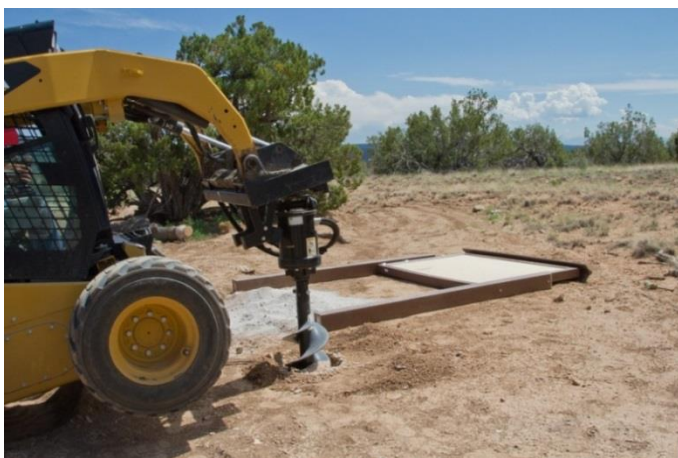
Installation of new informational kiosk at the trailhead for the Old Road trail in TA-70.
